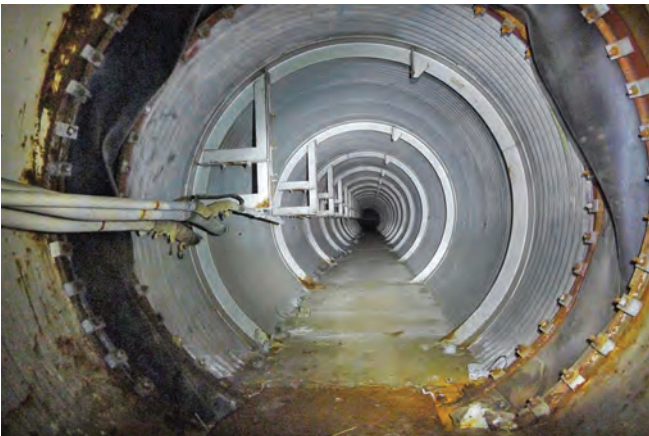
View of the LAUT. This section connects the cable entry structure with the PEUT further around the bunker
